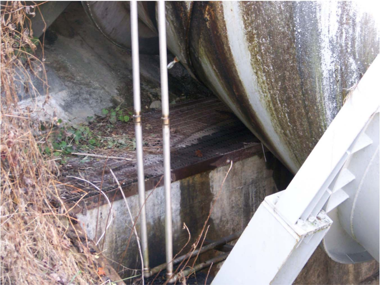
Unit 1 Penstock Butterfly Valve Foot and Oil Leakage into Storm Drains
